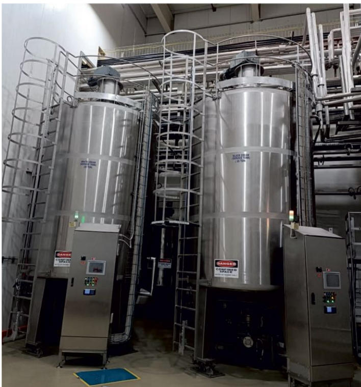
CHOCOLATE STORAGE AND HANDLING SYSTEM
